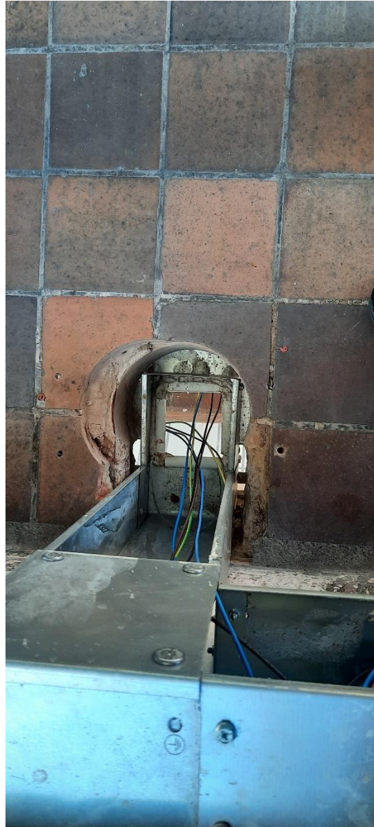
Figure 6 - Exposed wiring at Purser House
