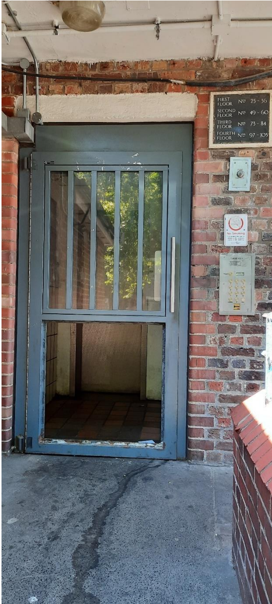
Figure 5 - Broken door at Purser House
