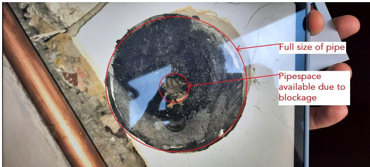
Figure 4 - A resident of Holt House showing pipe blockage photo on their iPad.
