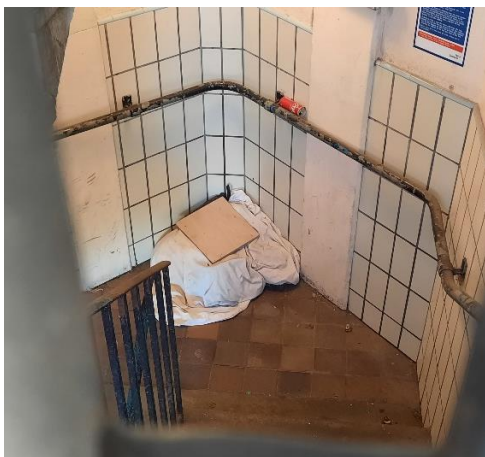
Figure 7 - Rubbish in stairwell
